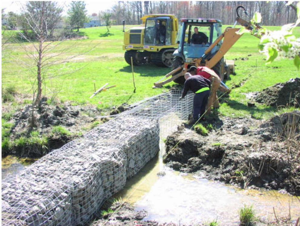
Figure 3. A barrier of gabion baskets spreads stormwater runoff in the basin (Photo Credit: Craig McGee, Camden County Soil Conservation District).
