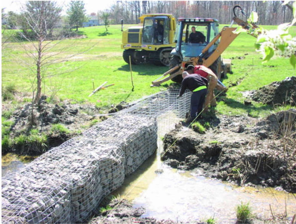
Figure 3. A barrier of gabion baskets spreads stormwater runoff in the basin (Photo Credit: Craig McGee, Camden County Soil Conservation District).
